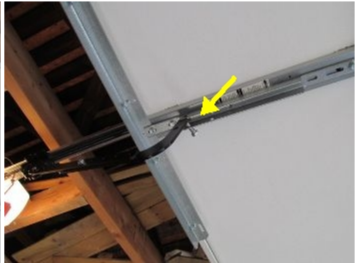
Loose bolt at left door
