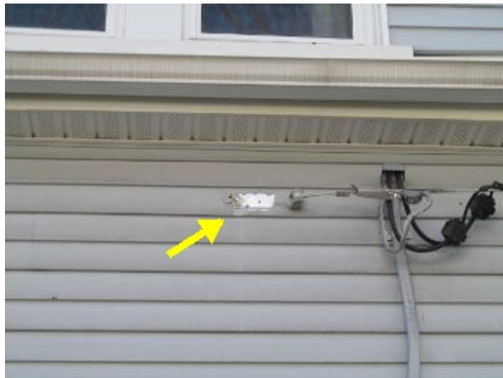
Damaged section of vinyl siding observed
