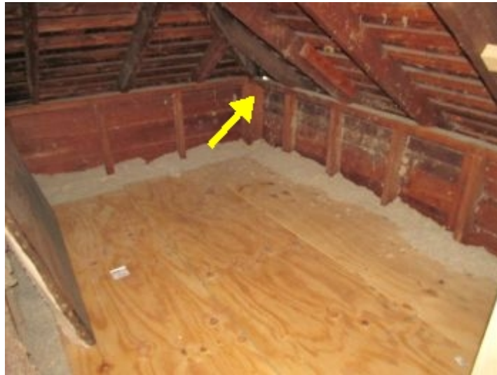
Gap in fascia observed through attic access, this should be corrected to prevent rodent entry
