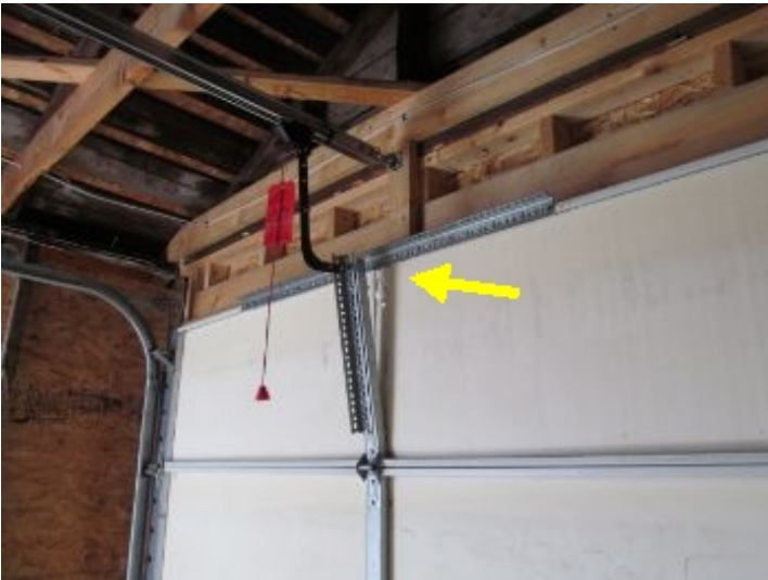
Damaged top door panel panel at right side door
