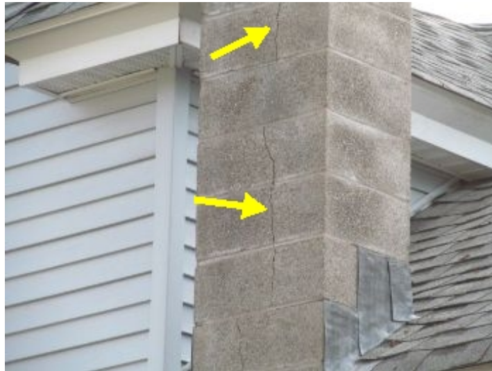
Cracked block observed
