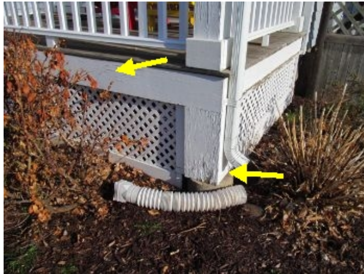
Weathered at front porch, recommend re painting to prevent damage to wood
