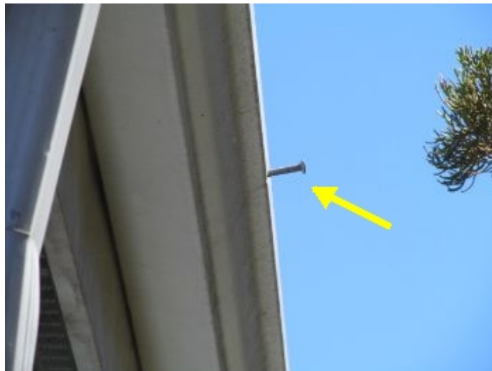
Loose gutter nails at right side of garage
