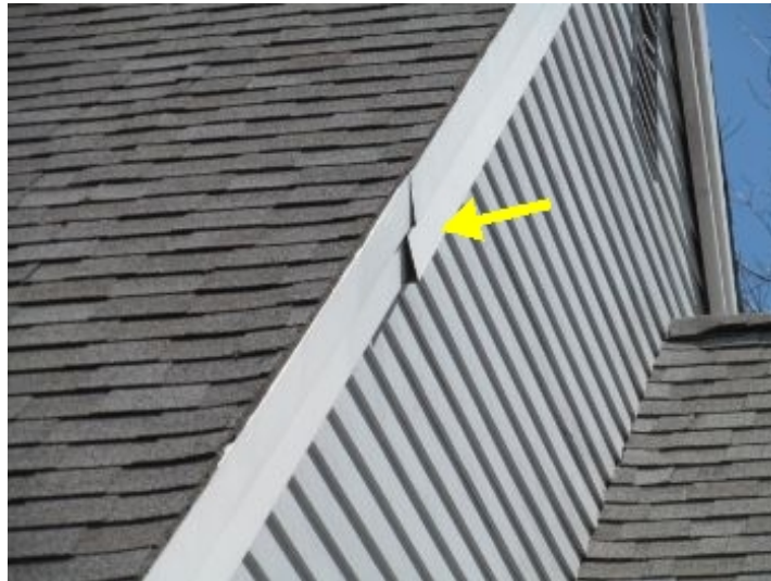
Loose fascia observed at right side rake trim
