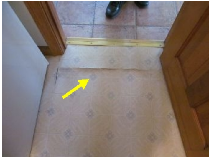
Cracks observed in concrete floor
