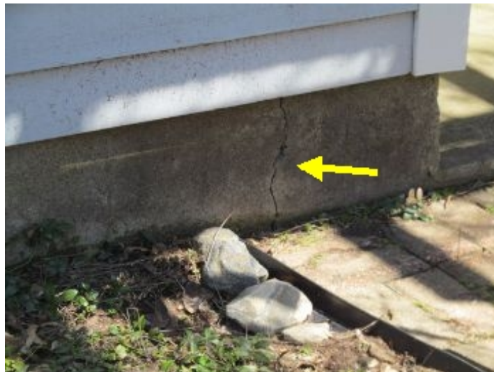
Crack observed at right side rear corner
