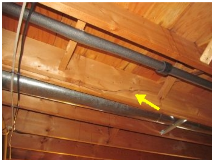
Broken joist observed but appeared to be sound because of additional joist along side
