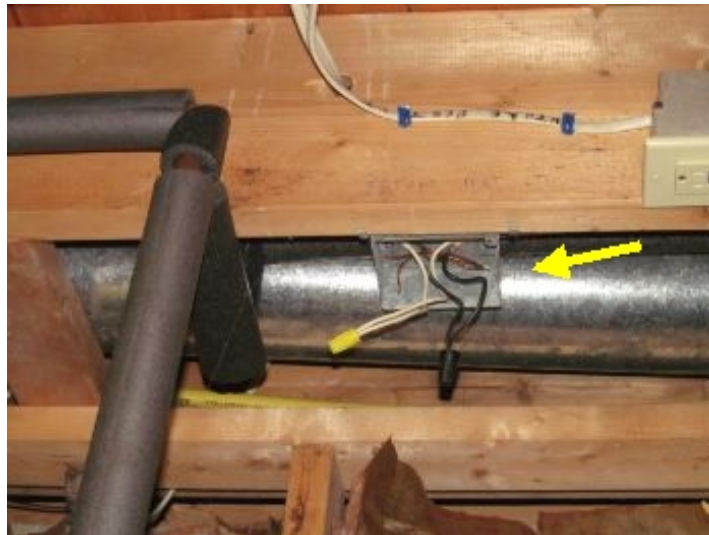
Missing electrical box cover
