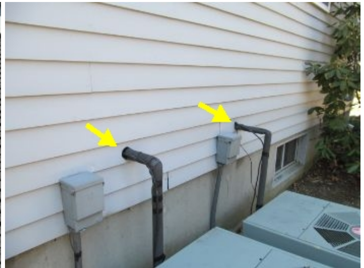
Recommend sealing holes & gaps around wall penetrations with polyurethane caulking
