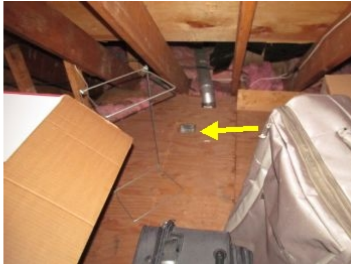
Missing electrical box covers
