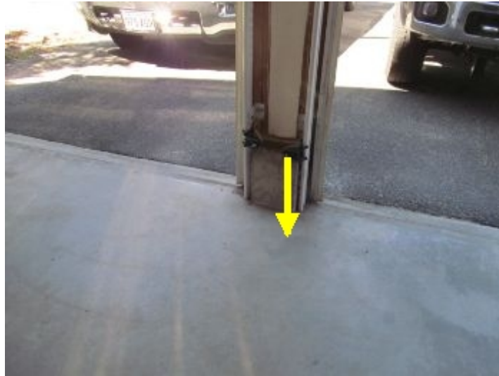
Electric eye units too high, manufacturers recommend 6" from floor or less
