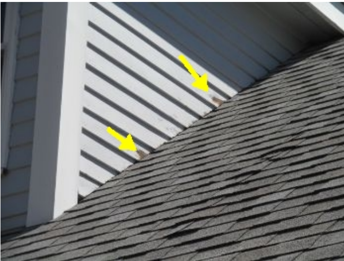
Deteriorated at roof contact points
