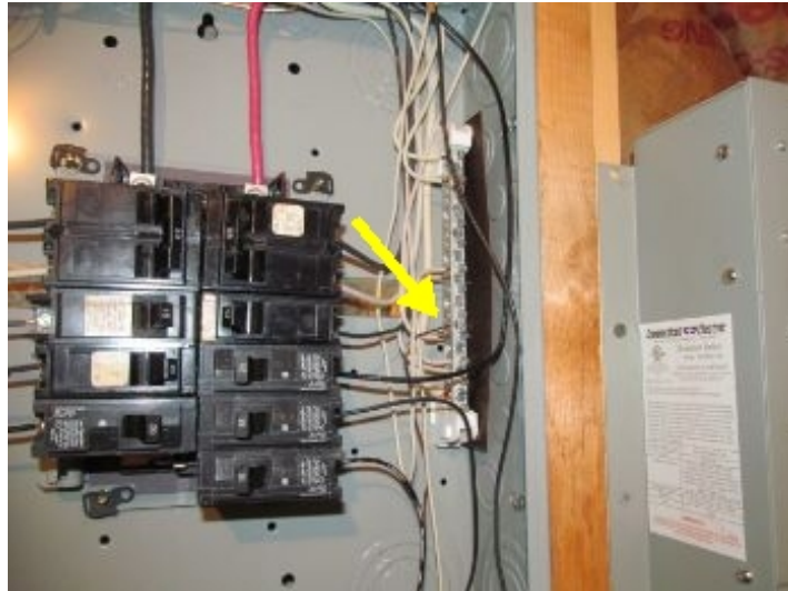
Ground wire attached to neutral bus in sub panel
