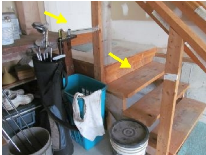
Garage stairs not child safe, require proper railings
