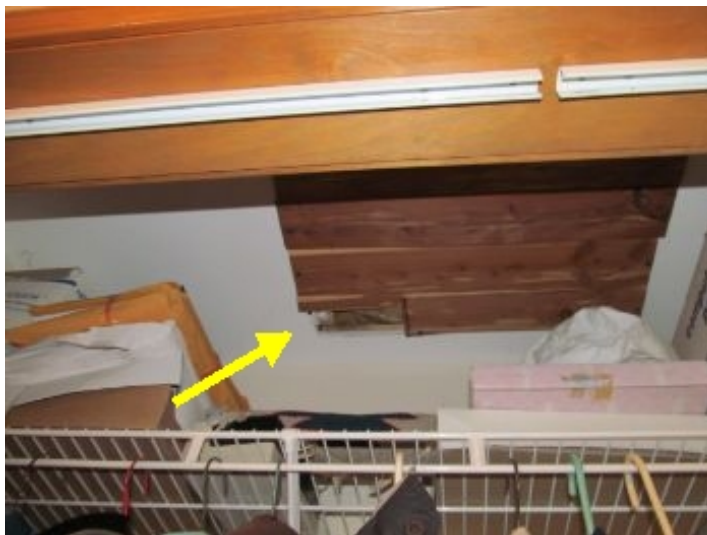
Recommend insulating and air sealing old scuttle cover
