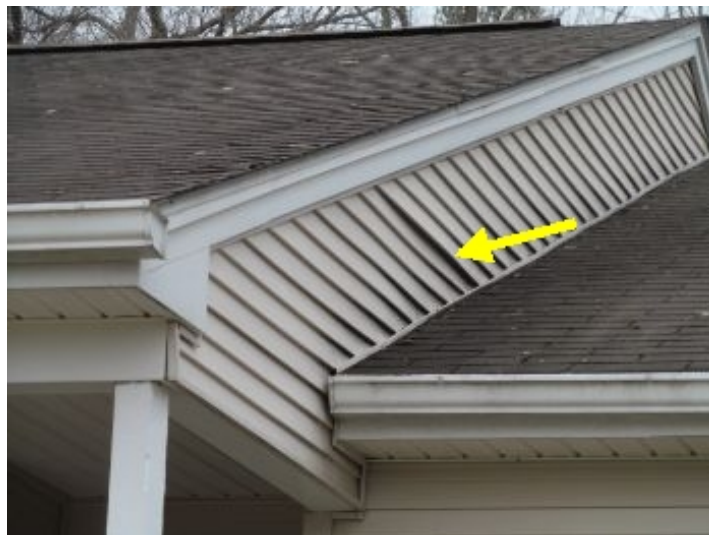
Loose siding observed
