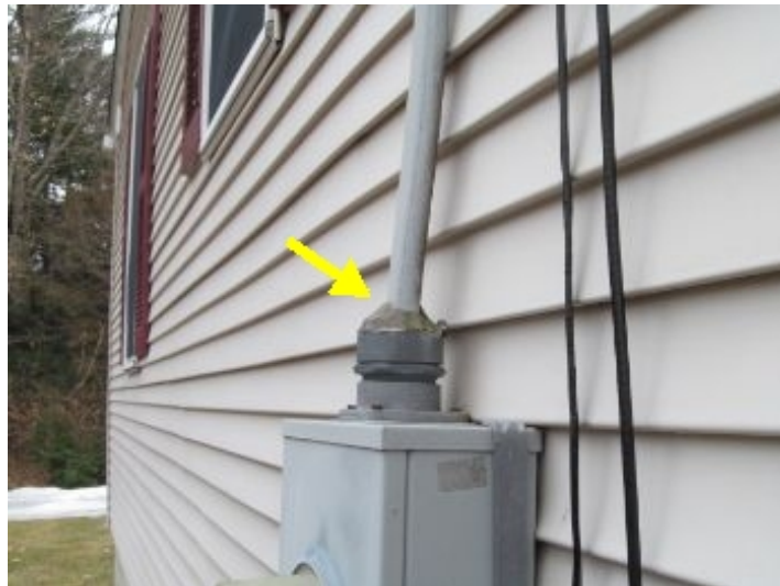
Cable entry into meter socket needs to be sealed properly
