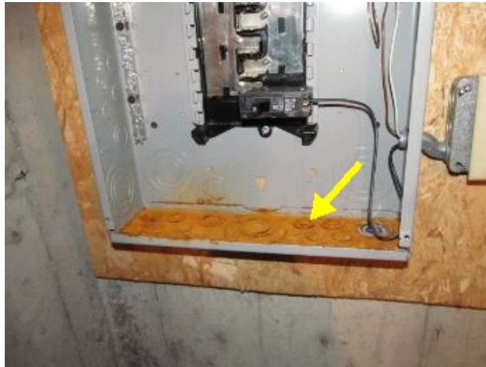
Evidence of water in panel
